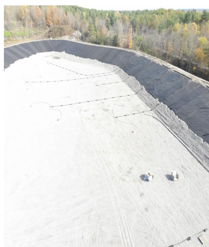
Third Lagoon cell pictured Fall 2021. Now fully operational.
